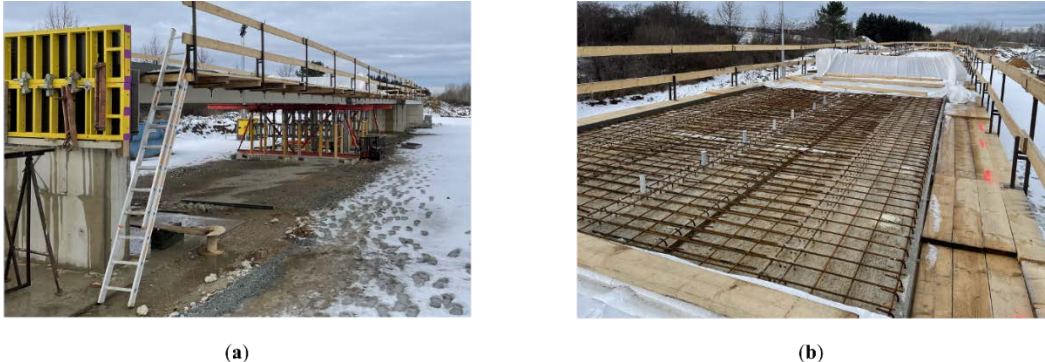
Figure 2. The openLAB in the construction phase shortly before concreting the additional in situ concrete in January 2024. (a) View of the entire structure; (b) view of the construction status of the superstructure.
