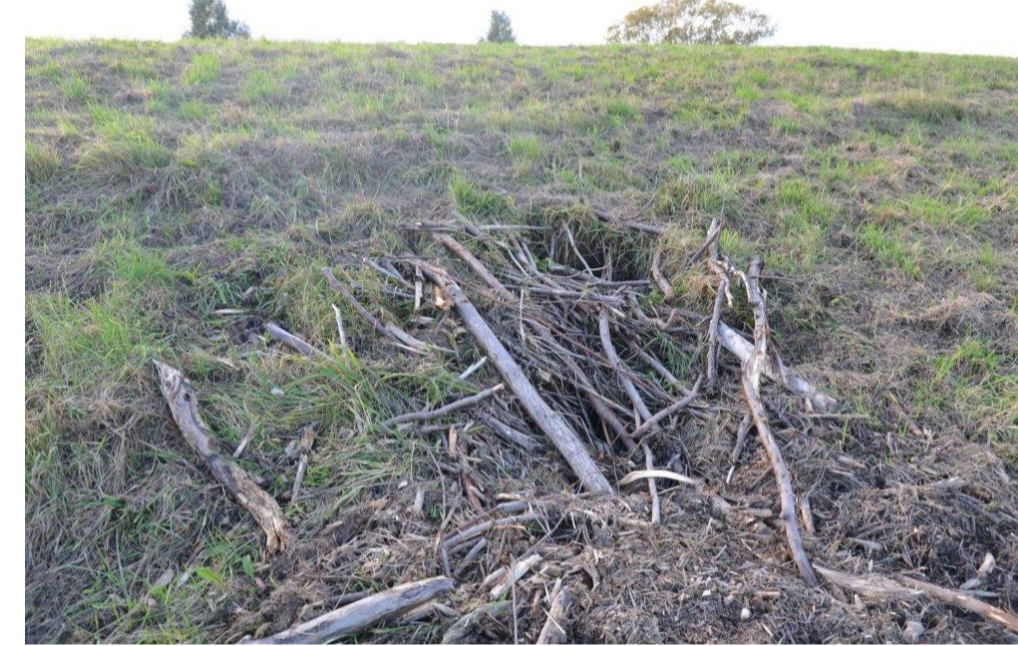
Figure 2 – Entrance to a beaver-caused cavity system in a river levee (Photo: LfU Brandenburg)
