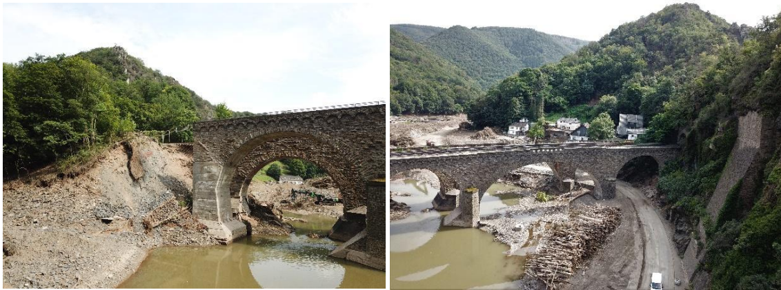
Figure 12: Photo of the abutment region of the double bridge, August 13 th , 2021. Left: Washed out abutment area, Right: bridge abutment area intact and connected to adjacent rock slope
