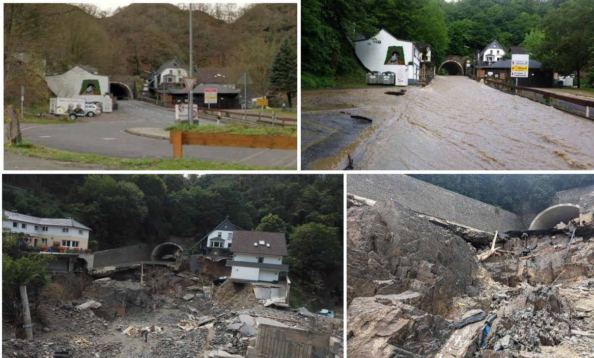
Figure 8. Top left: Google Earth/Maps Street View of the Altenahr tunnel from May 2021; top right: photo during the June 2016 flood event (Source: https://www.altenahr.de/index.php?id=26&publish[id]=9709&publish[mode]=overview&no_cache=1#18 ); bottom: photos by the reconnaissance team after the 2021 flood, August 2021 (50.5165261, 6.9975355)
